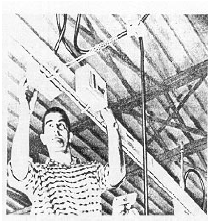
Figure 76—Installation View of Small Plug-in Busway Showing Individual Circuit Breaker Power Tapoff and Flexible Bus Drop Cable
