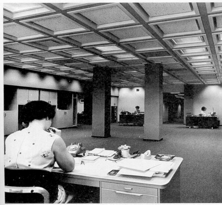
Figure 129—Two Foot by Two Foot Luminaires Containing U-Shaped Fluorescent Lamps
